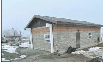
The rebuilt Bridgeport wastewater treatment lab was scheduled to be occupied and operating by the end of January.
